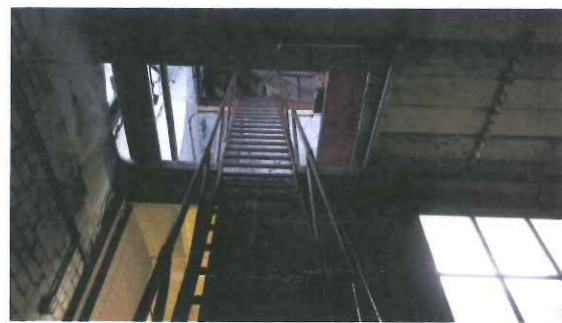
2.) View from base of ladder A showing temporary scaffolding to right hand side. Ladder length 6590
