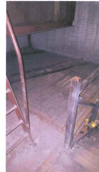
4.) Showing base of ladder A next to stairs
